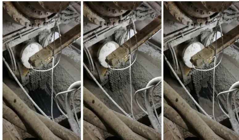
Figure 14. Muck discharge at the screw conveyor with conditioned material forming a plug in the screw with 4 bar of confinement pressure in the excavation chamber (no fluidification).
